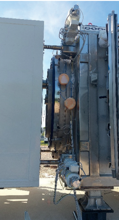
LH2 storage system
